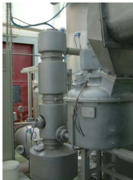
At present. Feed tank and drying chamber
