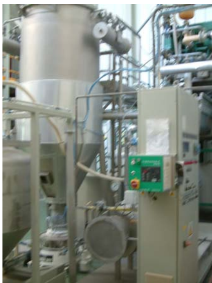
At present. Bag filter and control screen
