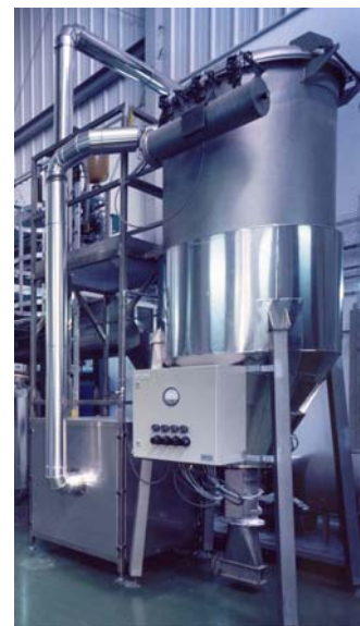
Installation after mounted
